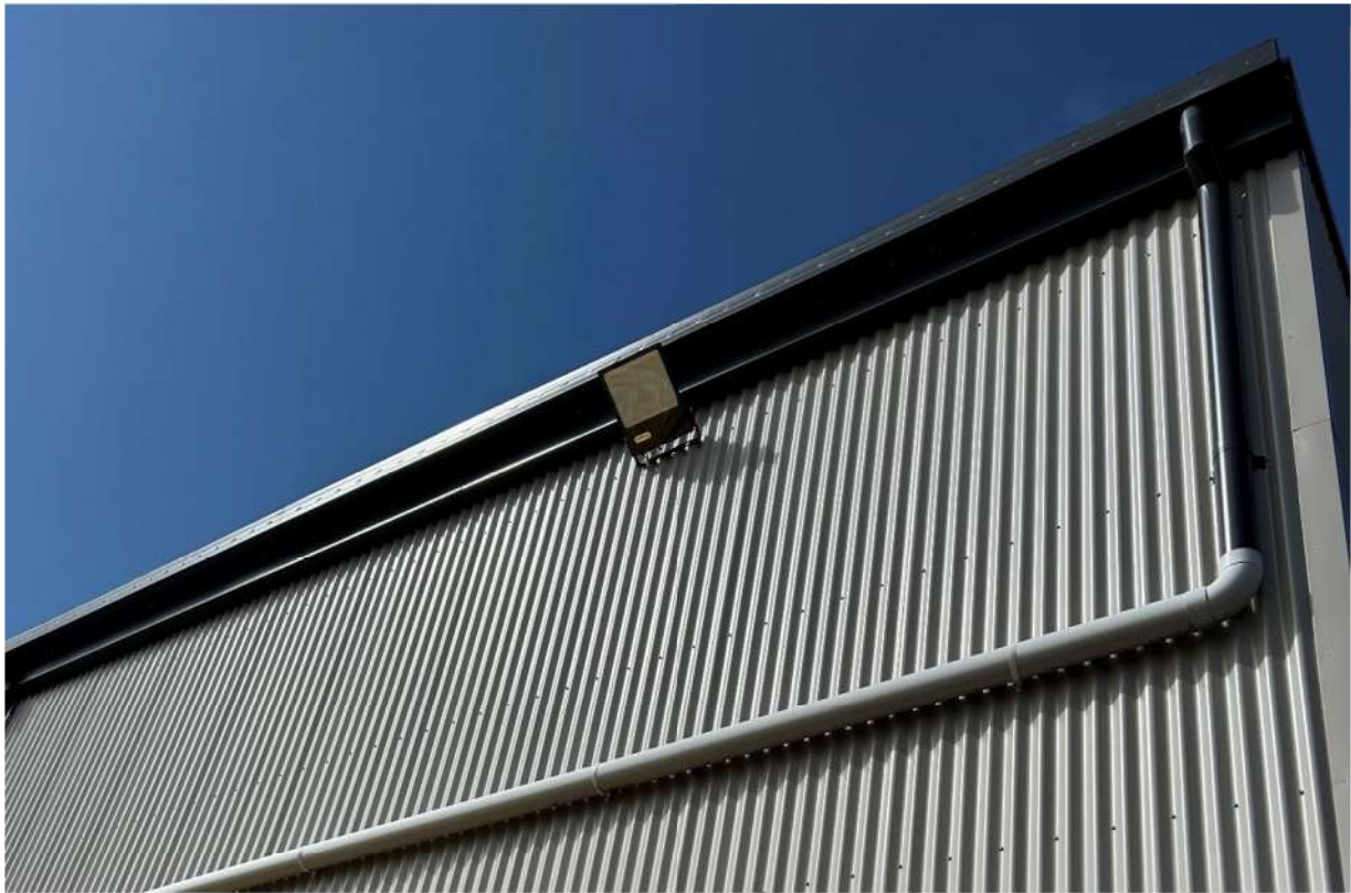
Plate 9 – Lighting on O&M building
