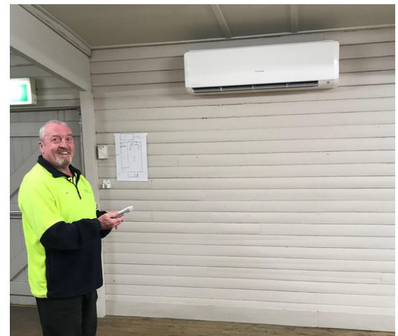
BJCE Australia recently funded the installation of a reverse cycle air-conditioning unit at Grabben Gullen Community Hall.
